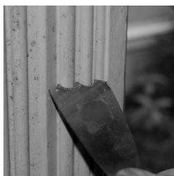
Custom scraping tool fabricated by Bill Hole to match historic casing molding for ease in paint removal
