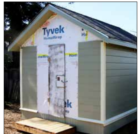
The new garden shed under construction with siding and a temporary door. Heritage Society photo.
