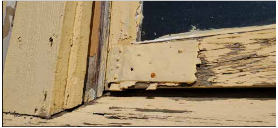
A metal bracket holds a badly deteriorated window together prior to repairs. B. Seivertson photo.
