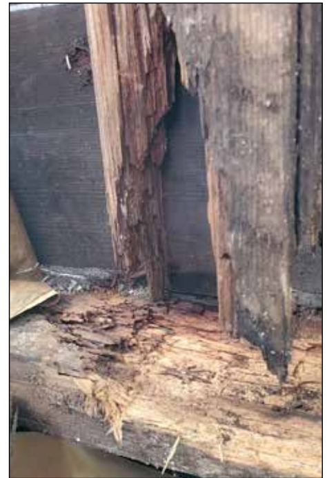
Water intrusion damage to a wall stud next to a window. B. Seivertson photo
